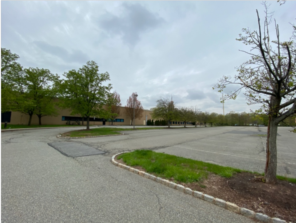
Figure 34: One of the dead landscaping trees and patched area of site
