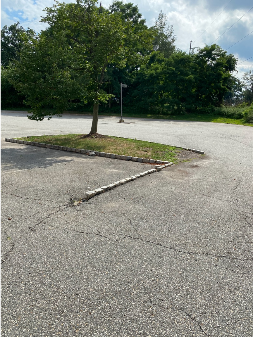
Figure 39: Signs of erosion
