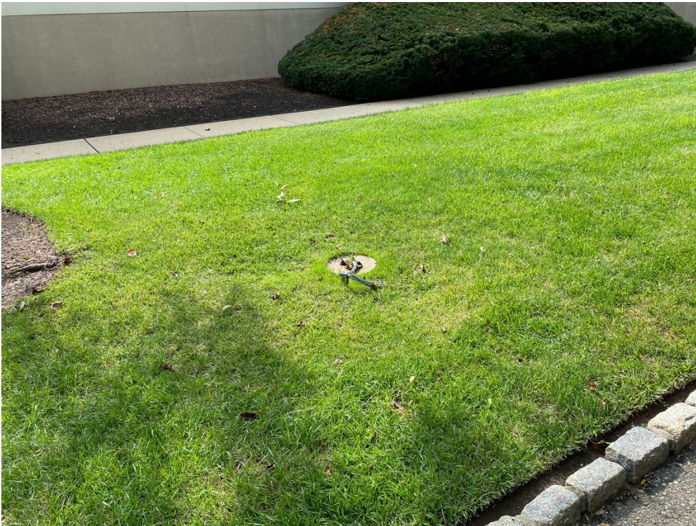
Figure 12: Missing pedestrian safety lighting
