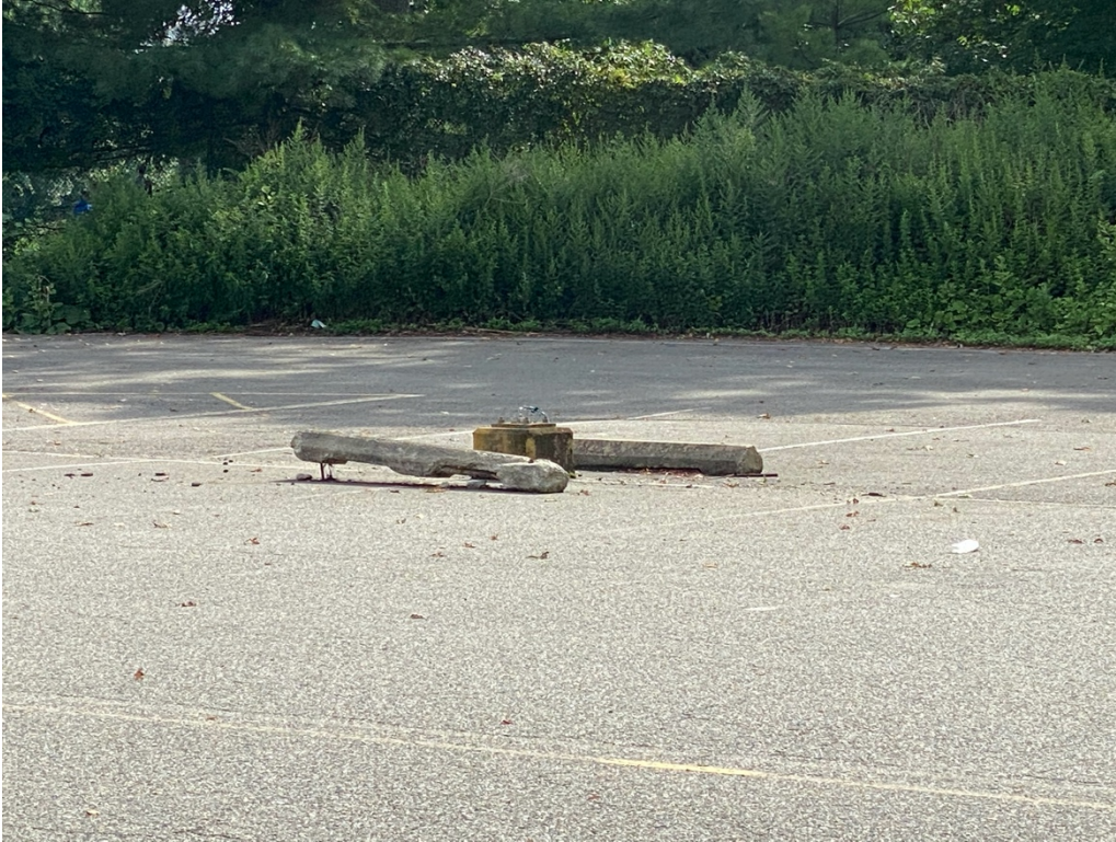
Figure 5: Missing safety lighting and damaged circulation controls
