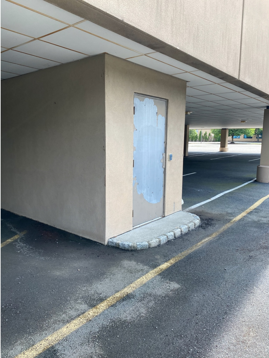
Figure 7: Deferred maintenance and chipping paint
