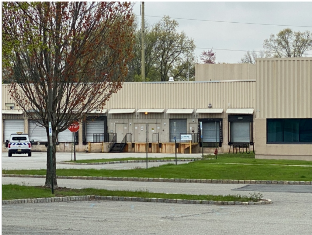
Figure 4: Undersized, deteriorating loading bays
