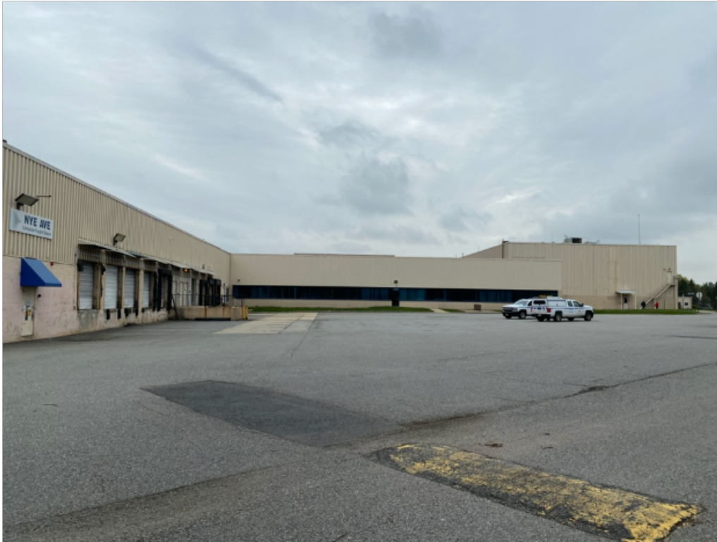
Figure 11: Damaged parking lot and one of the missing speed humps
