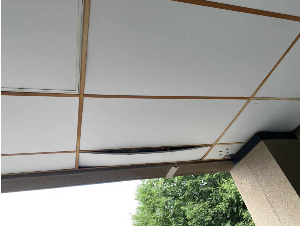
Figure 5: Bird nest in ceiling of indoor parking area
