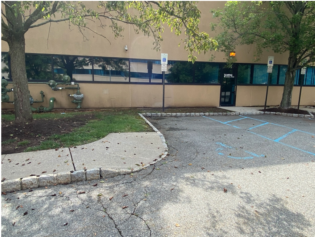
Figure 18: Inaccessible ADA ramp (2)
