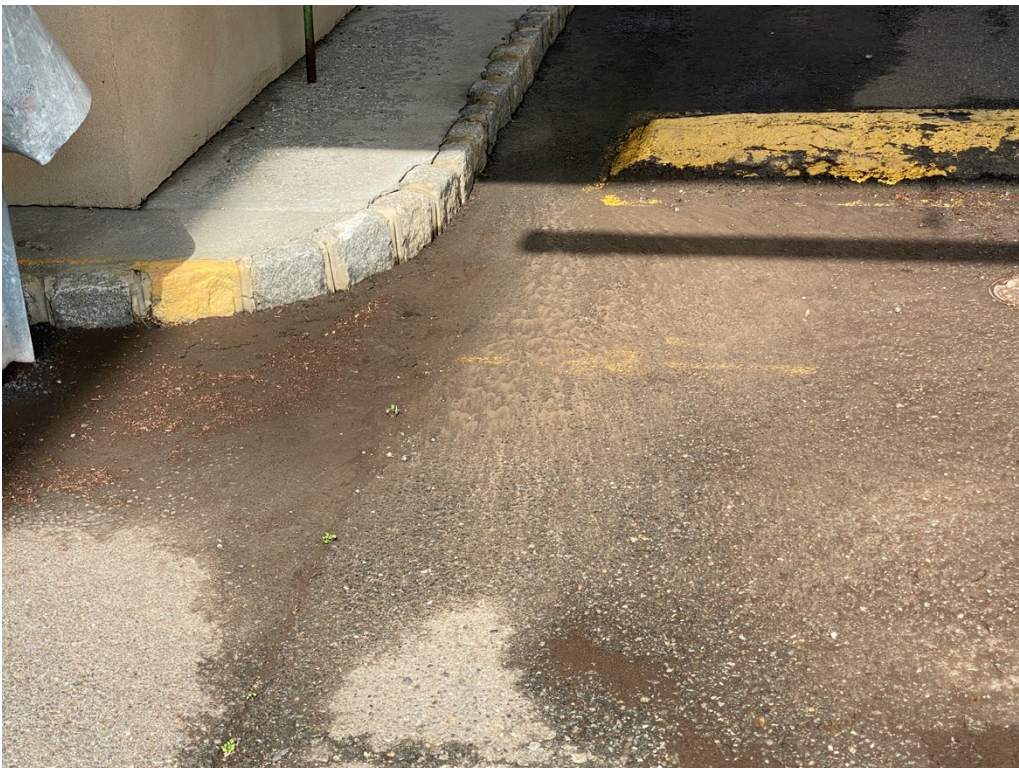
Figure 6: Pooling stormwater and signs of erosion
