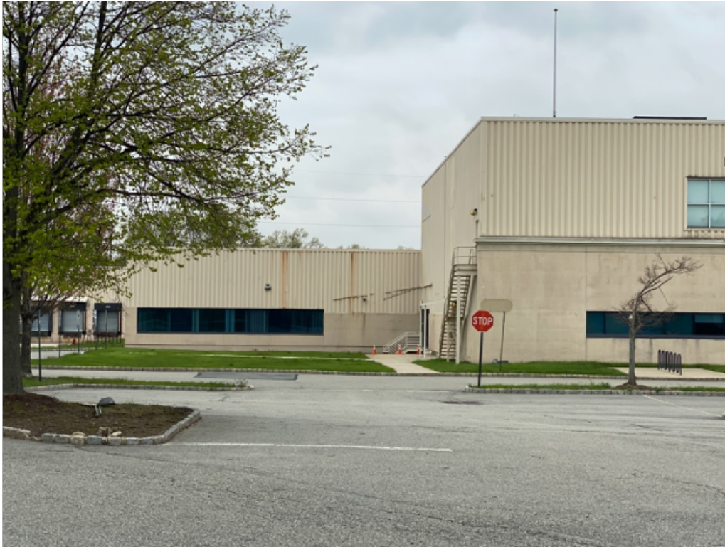
Figure 8: Water damage and deferred maintenance
