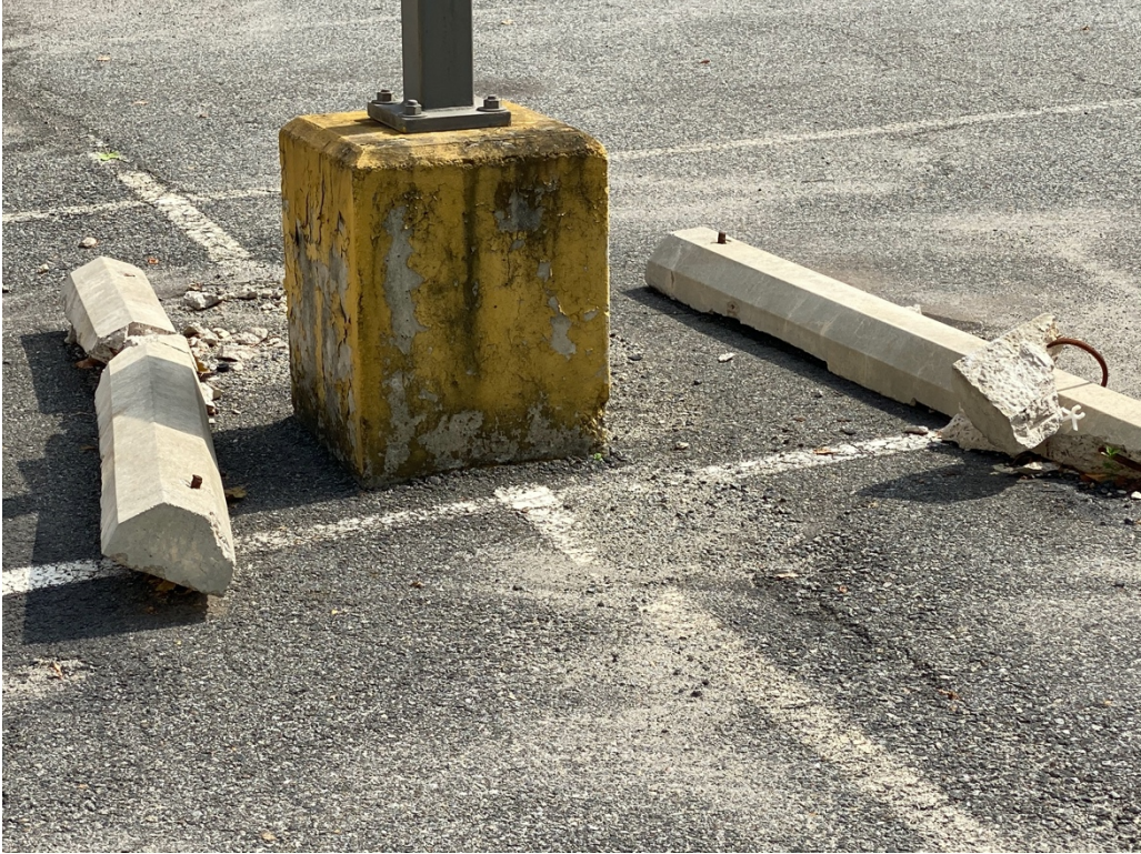
Figure 2: Damaged circulation controls
