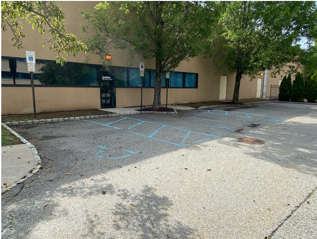
Figure 26: Undersized ADA accessible parking spaces
