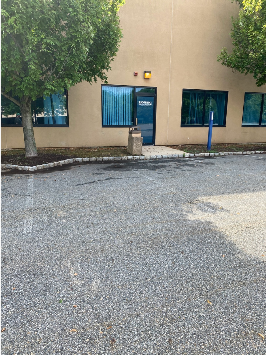
Figure 19: Non-ADA compliant ramp
