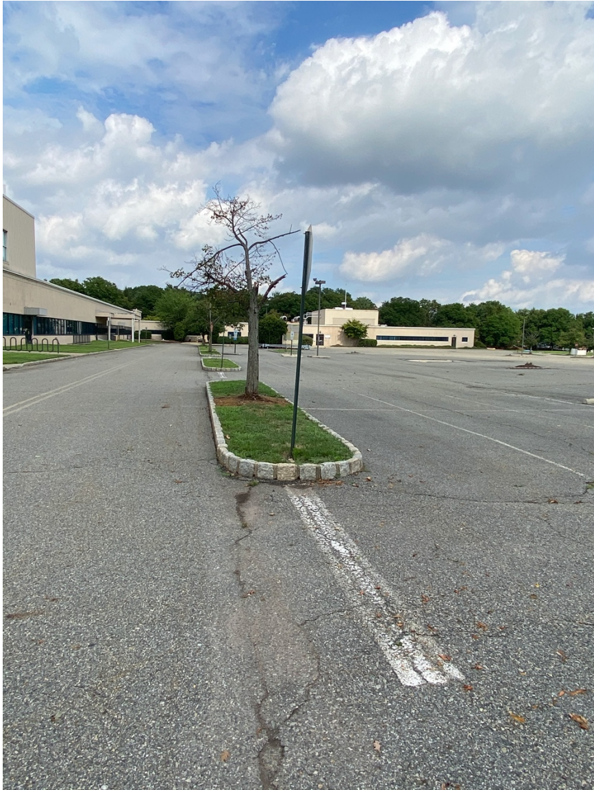
Figure 20: Lack of pedestrian controls from ADA-required accessible parking spaces
