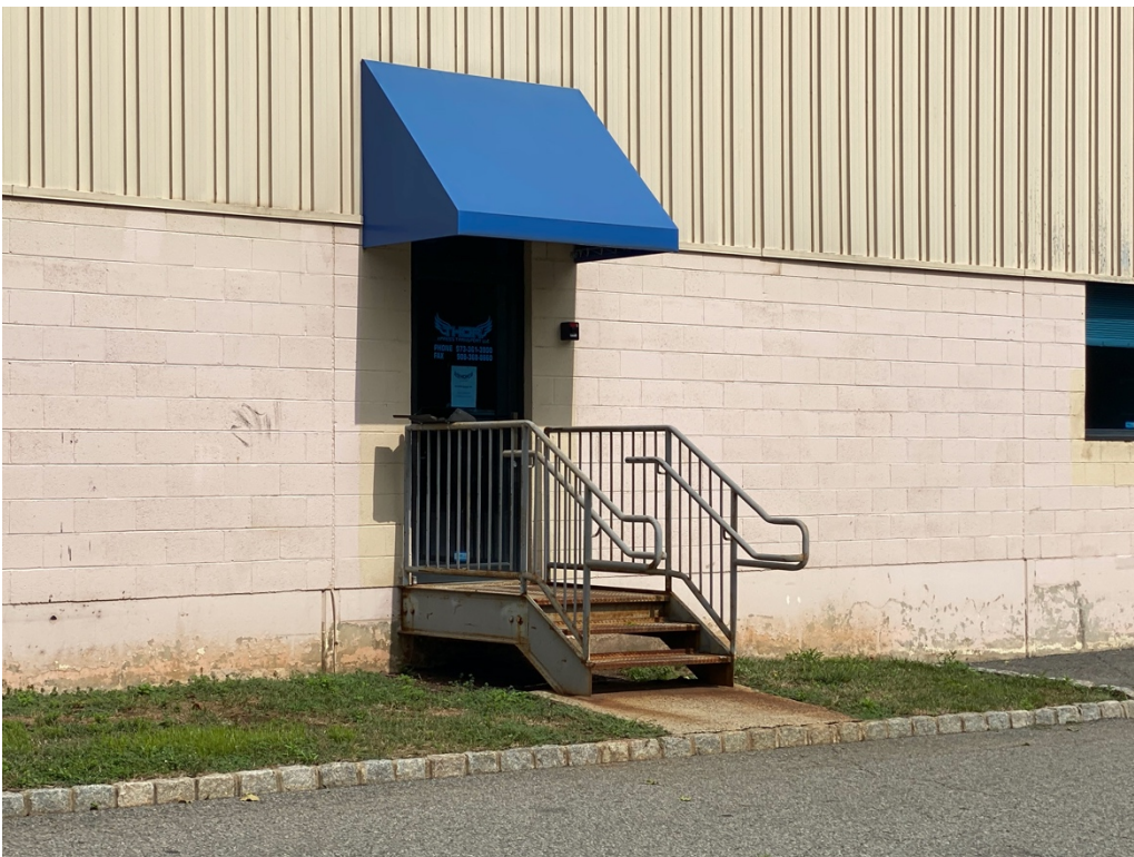
Figure 9: Rusted, broken stairs
