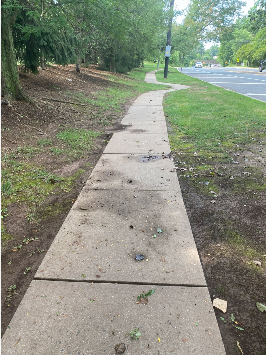
Figure 38: Signs of erosion from site
