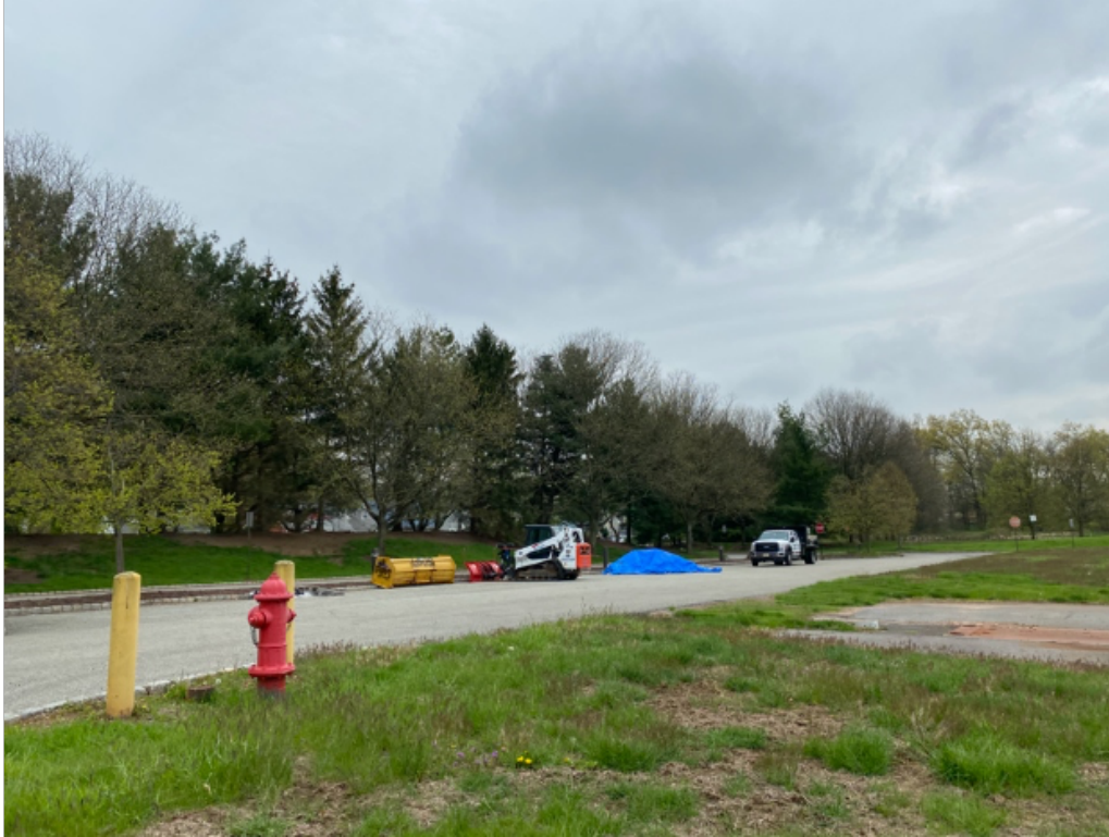
Figure 9: Missing curbing, deferred maintenance, storage on-site and damaged asphalt
