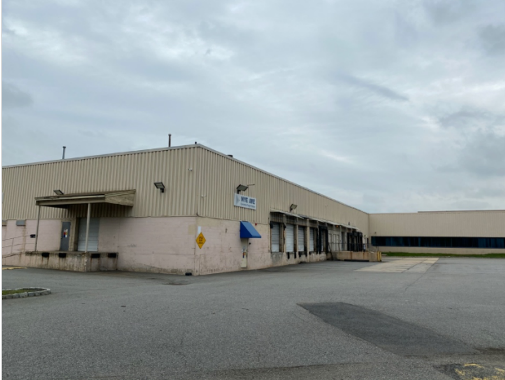
Figure 3: Damage to foundation and façade
