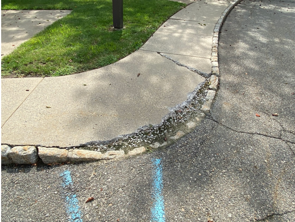
Figure 17: Inaccessible ADA ramp (1)
