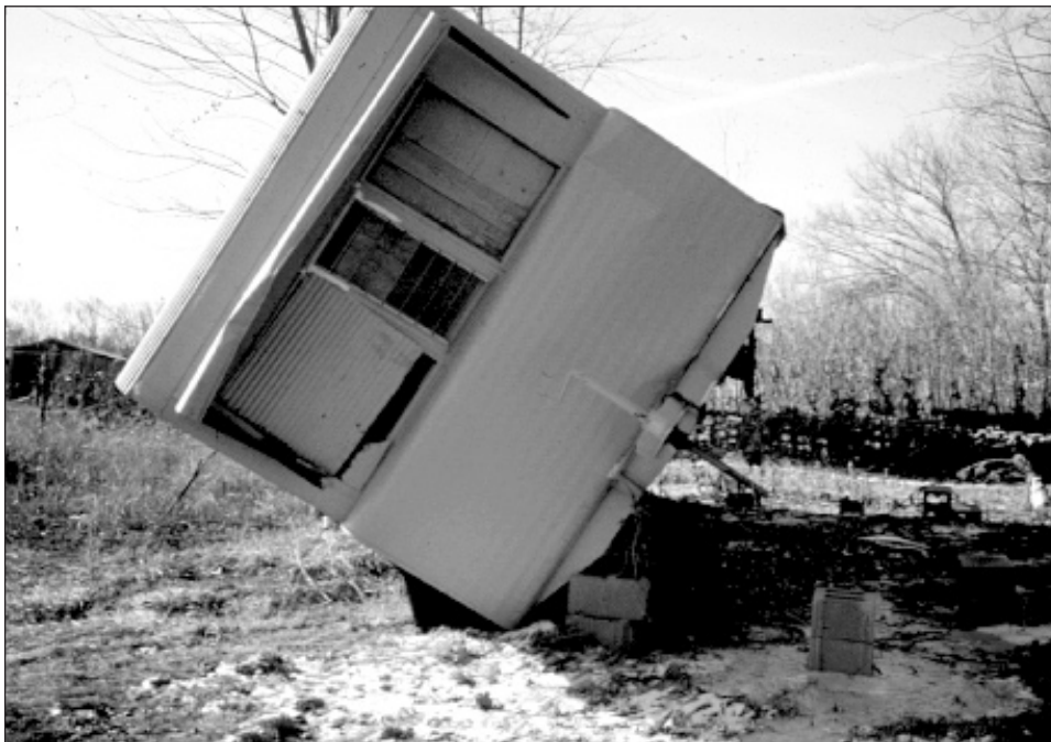
Figure 7-8. Failed foundation system that used masonry piers.
