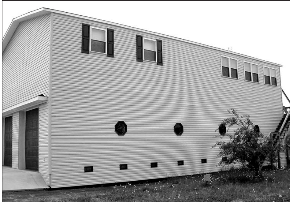
Figure 8-1. A manufactured home elevated on a perimeter foundation wall. Although it appears the openings are too high, the bottoms of the openings are less than 1 foot above the top of the interior slab.
