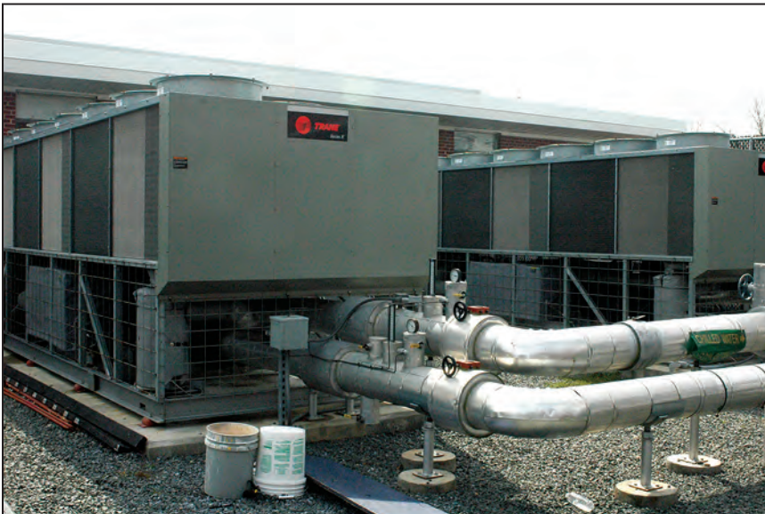
Figure 5-3. Air-Cooled rooftop chiller in Georgetown, Delaware.
