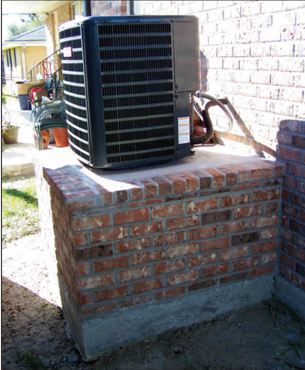
Figure 3-1. Air conditioning compressor elevated on a pedestal.
