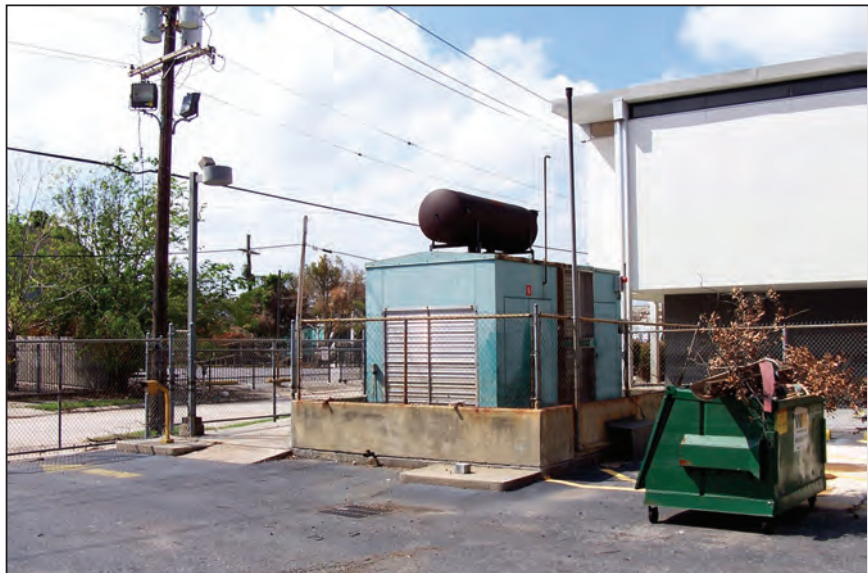
Figure 3-3. Protective flood barrier surrounding shed housing back-up power generator.
