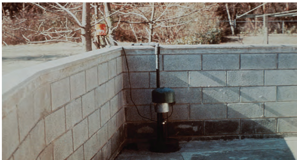
Figure 8-6. Small patio floodwall with sump pump.
