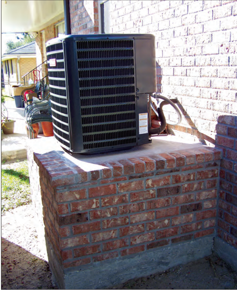
Figure 9-1. Air conditioning / heat pump compressor mounted on a brick pedestal outside an elevated home.
