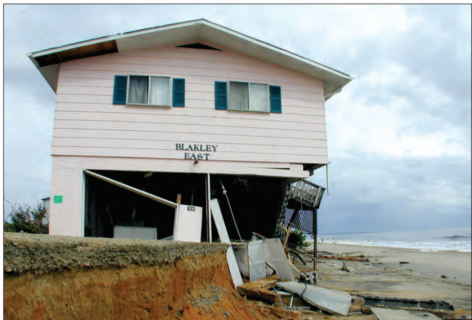
Figure 2-4. The extreme impact of large, fast-moving waves, combined with the removal of supporting soil by erosion and scour, can have devastating effects on buildings exposed to coastal flooding. Hurricane Floyd destroyed this home along the coast of North Carolina in 1999.
