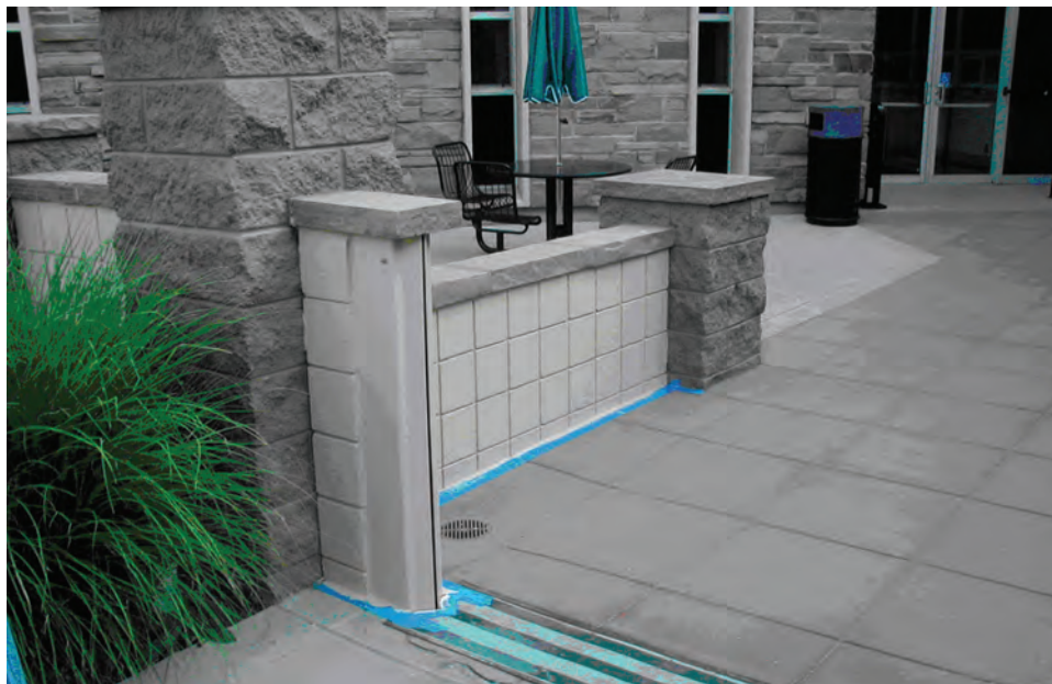
Figure 8-5. The City of Boulder, CO, installed a “pop up” closure to this floodwall at a City office building subject to flash floods. The closure floats up into place automatically when the site is flooded.
