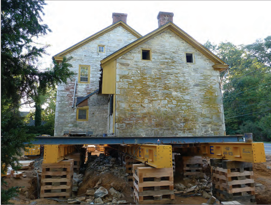
Figure 6-5. Hydraulic jacks lift the structure, and the home is separated from existing foundation (photo courtesy of Wolfe House Movers).
